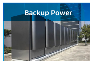
Future-proof, reliable and clean energy reserves
